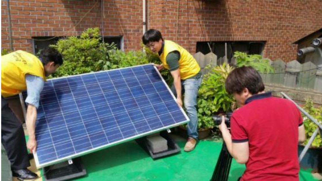
Civic activists install a solar panel on a rooftop. (Source: Seoul City)
