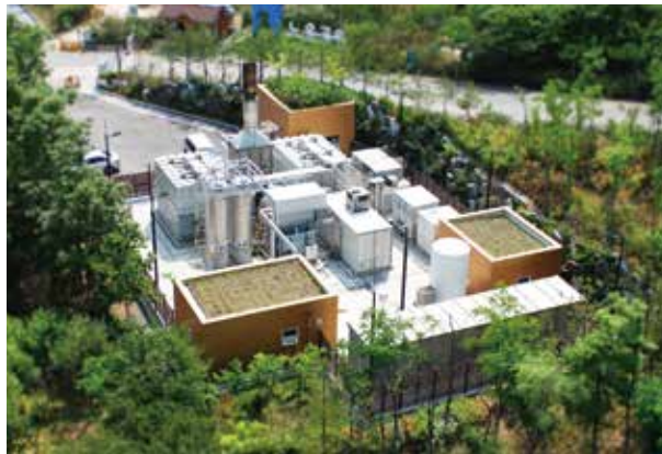
MCFC-type fuel cell station in Sangam (2.4 MW)
