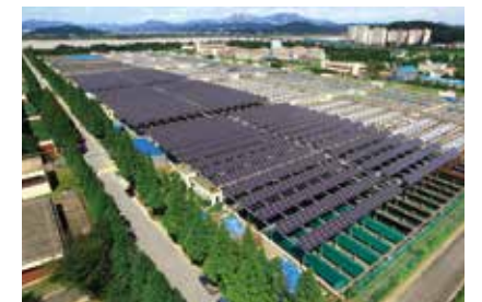
Solar panels at Seonam Sewage Treatment Center
