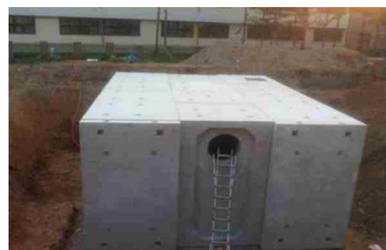
Rainwater Recycling Facility in a Park
