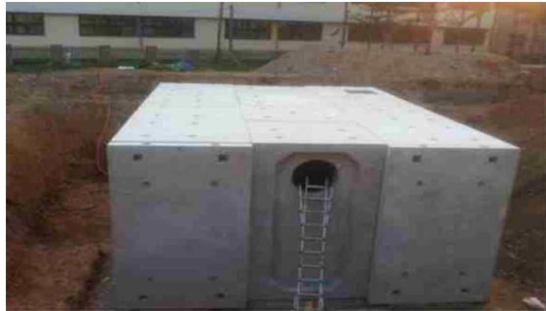
Rainwater recycling facility in a park
